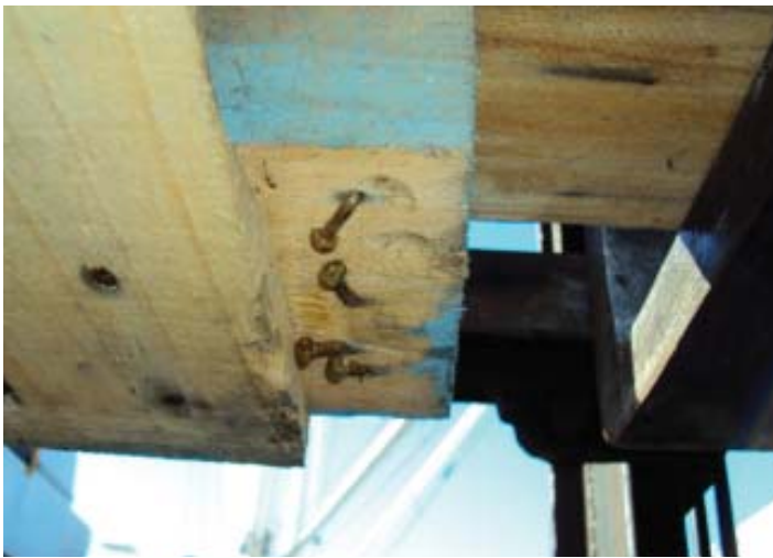
Flat rusty nails
